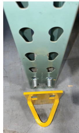
No Anchor Bolt On
